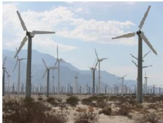
Fig.(2) a modern wind farm
